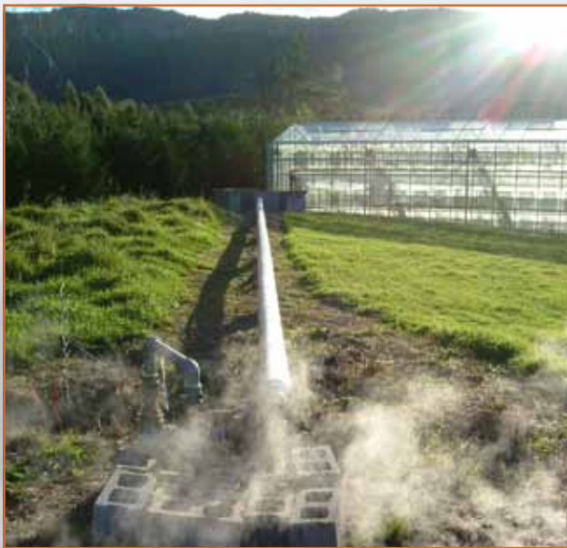
This geothermal bore produces 100°C water that is fed through a heat exchanger, heating water circulated in an internal closed heating system.
